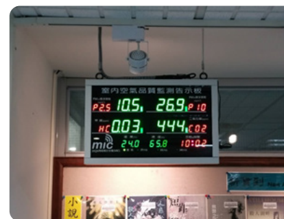
Indoor air quality real-time monitoring panel
